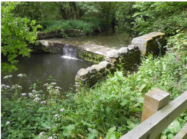
Figure 5 – safety fence at the left bank (to be replicated at the right bank until urgent works can be completed)
