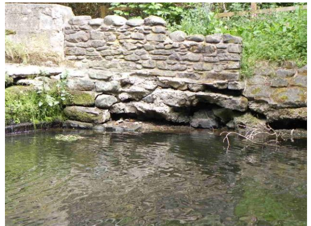
Figure 6 – section of new masonry at the left bank and area of erosion and undercutting.
