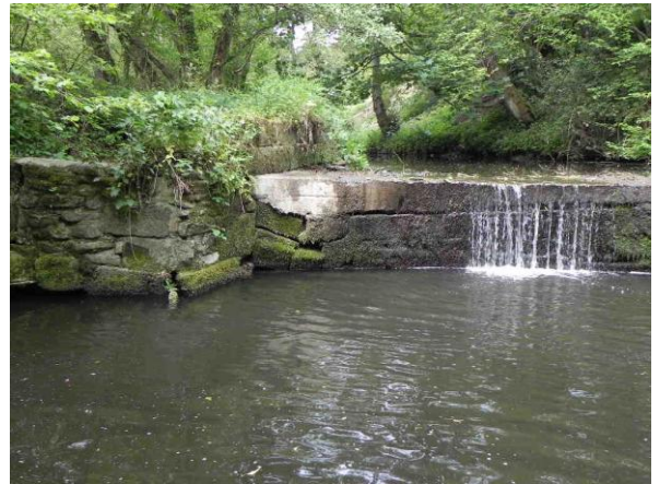
Figure 4 – the 'corner' to the left of the picture that is severely undercut below water level. The proposed notch would be roughly 2/3 of the weir height.
